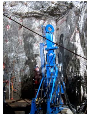
This is the first UE-24 drill to drill deep holes at Hoyle Pond in their newest Exploration Program
