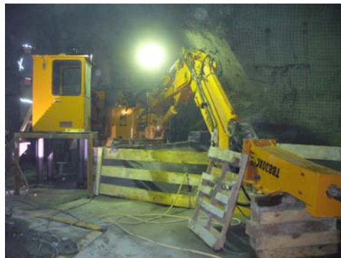
Bulk Zone Rockbreaker Assembly
