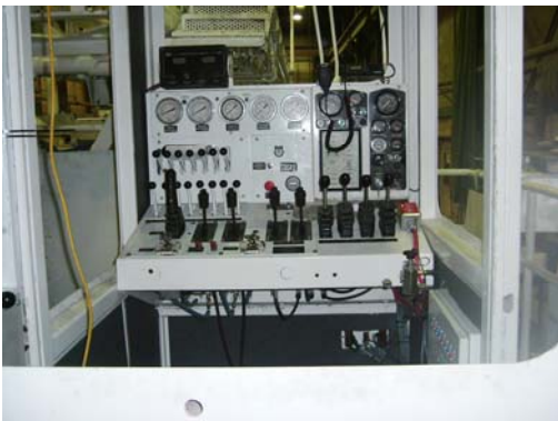
The cab was repaired to a "better than new" state by relocating the electrical panels and eliminating some unnecessary components, thus allowing more room for the operator.
