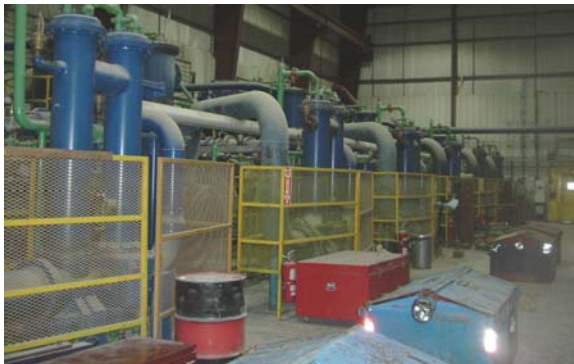
The old powerhouse compressors shown above have been sold and are currently in the process of being dismantled to make the long journey to their new home in Peru.
